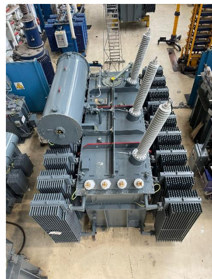
TR 40 MVA ONAN 150/20.8kV 6KV
